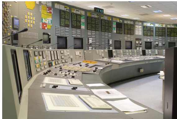
PPC, Security, Networks, Central Monitoring Systems
